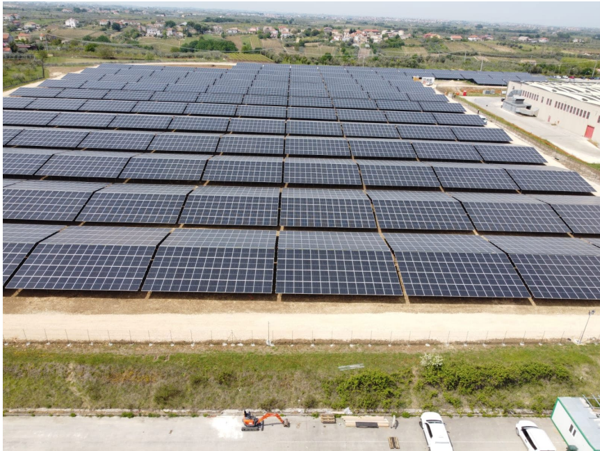
Ontex's new solar installation next to its plant in Ortona, Italy
