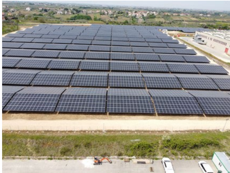
Picture: large solar installation for on-site power consumption at Ontex's plant in Ortona, Italy
