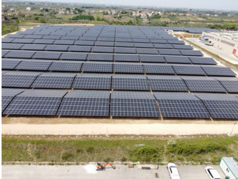
Picture: large solar installation for on-site power consumption at Ontex's plant in Ortona, Italy
